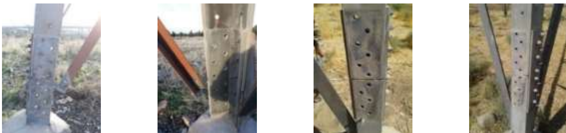
Fig. 1. Theft of the bolts of the connected members in the leg of the power transmission towers
